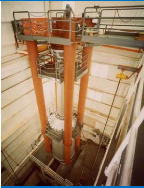
Fort St. Vrain Fuel Handling Machine
